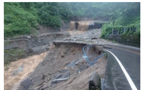
Ozo — Hakusan Shirakawa-go White Road The strong current of the river caused the road to collapse. Water services to the Ozo area were cut off due to damage to water intake facilities.
